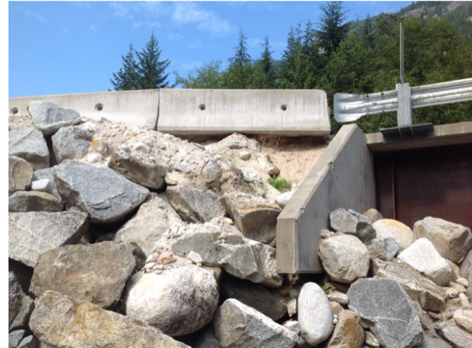
fill erosion under left upstream concrete barriers
